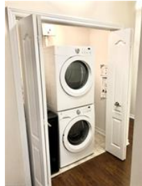
Laundry closet with water softener and hot water tank. Both owned.
